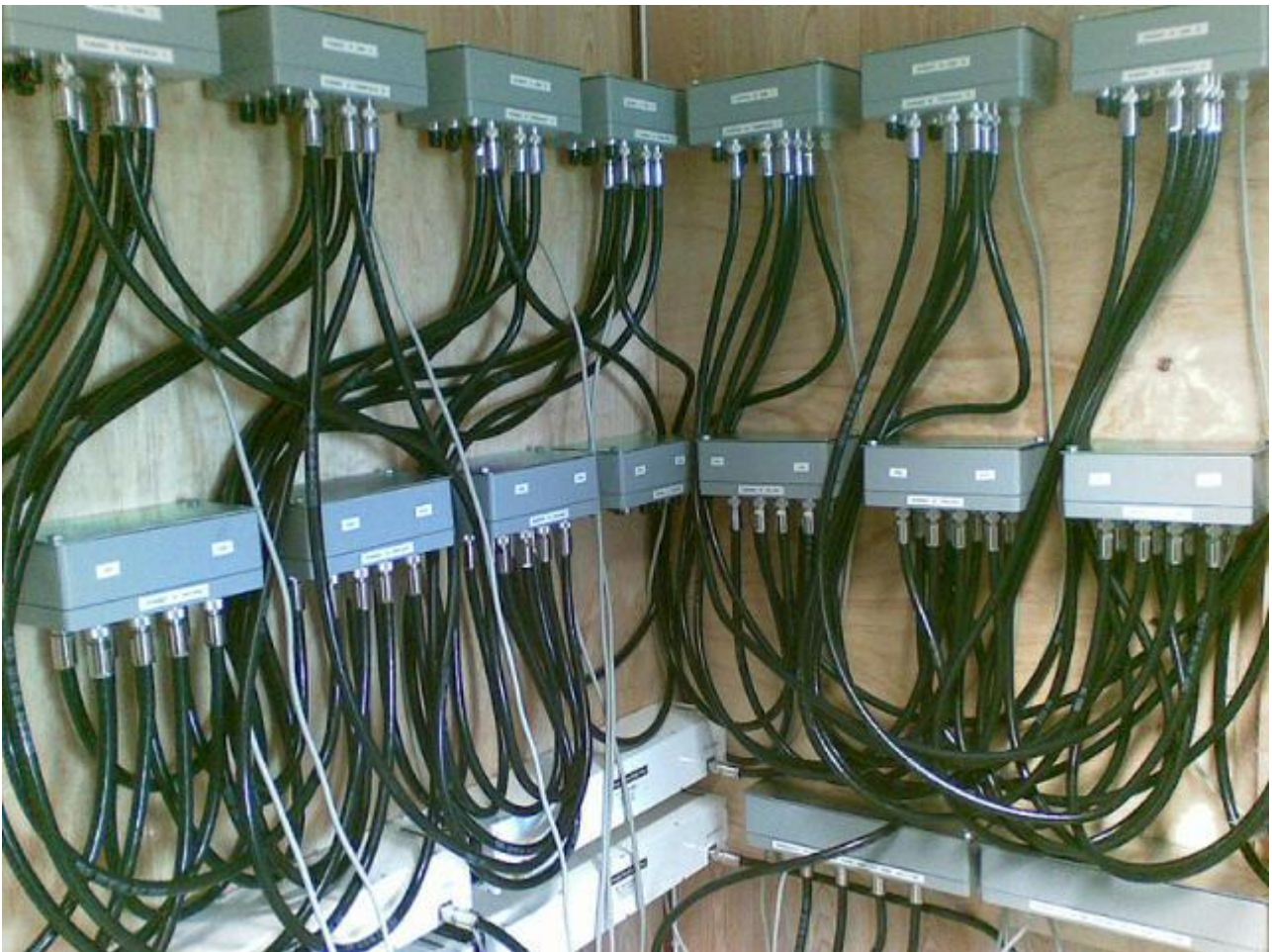
Post WPX CW cabling at OG8X (c.f. page 15).
